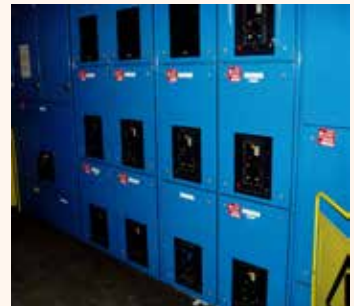
Obsolete Merlin Gerin Selpact ACBs
