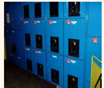
Obsolete Merlin Gerin Selpact ACBs
