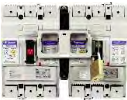
Slide Interlock Installed Between two MCCBs
