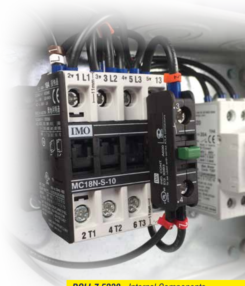
DOLI-7.5230 - Internal Components
