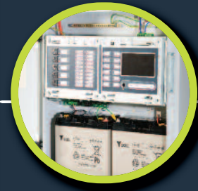
Up to 72 hours standby in standard cabinets
