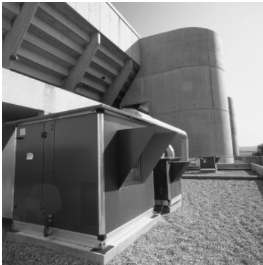
Air treatment application
