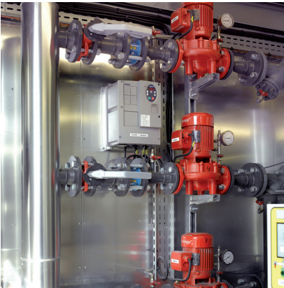
Air conditioning application
