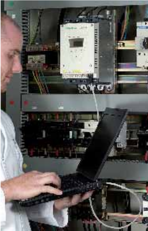
Commissioning the ATS 22 soft start - soft stop unit with SoMove lite setup software
