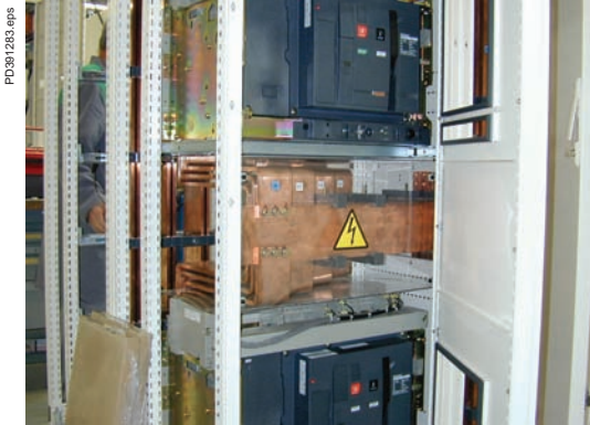
Source changeover system in the same cubicle.
