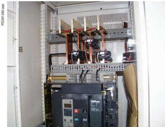
CT on vertical busbars.
