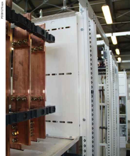
Dismountable vertical busbars.
