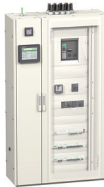
Power distribution switchboard.
