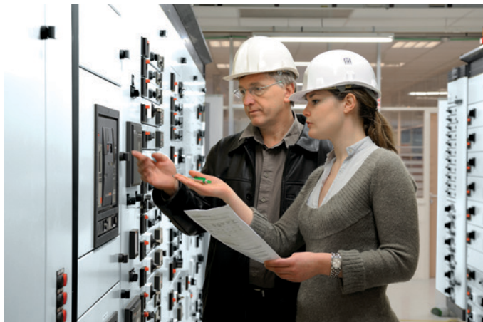
Motor Control Centre (MCC).
