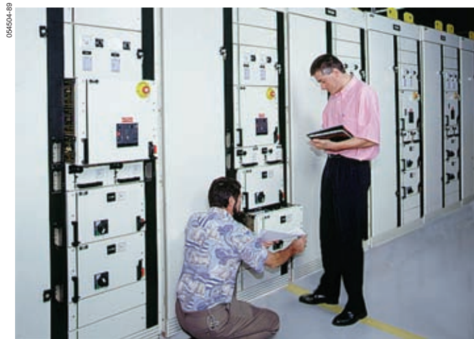
Motor Control Centre (MCC).
