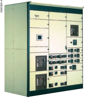
Main LV switchboard.
