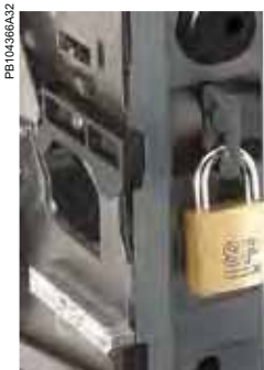
"Disconnected" position locking by padlocks.
