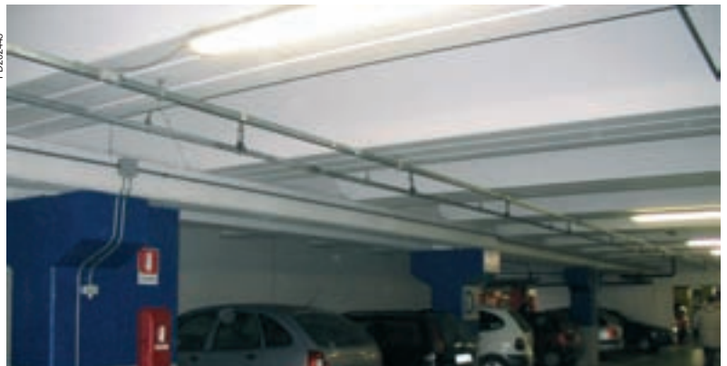
Canalis KBA supplying luminaires nearby sprinklers.
