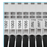
Clear terminal block identification Top large marker. Hand pre-marking before final marker installation
