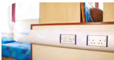
Odyssey trunking with Part M boxes installed at Old Swinford Hospital School, Stourbridge.
