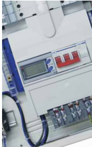
Metering fitted next to incomer within board
