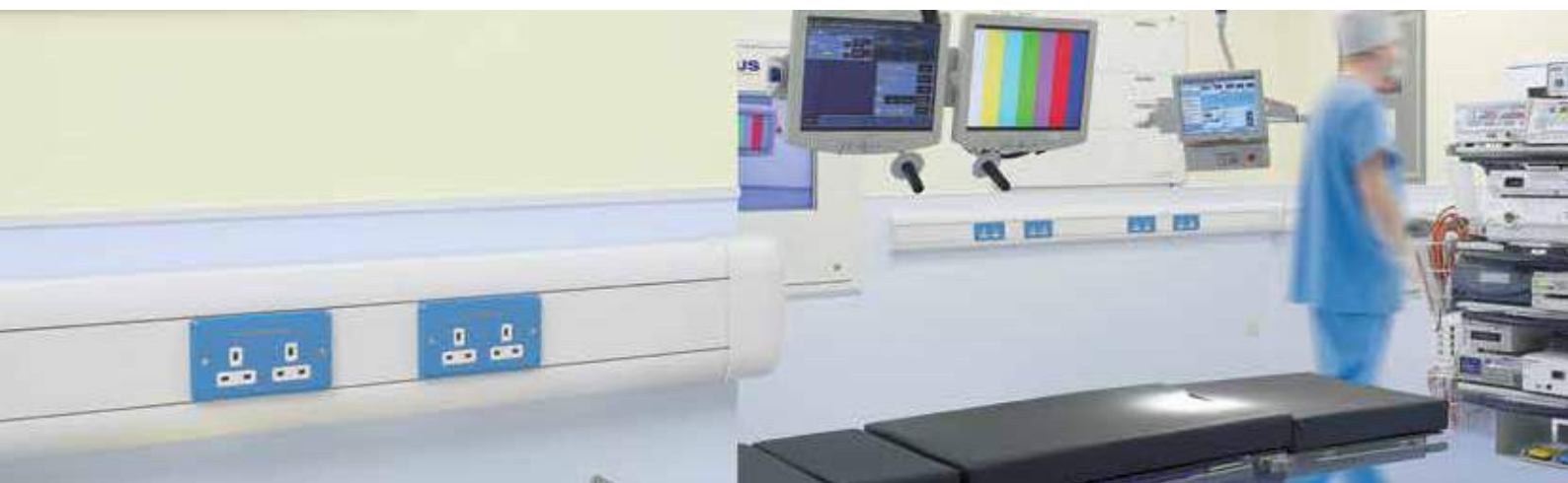
PRESTIGE 3D ANTIBAC BLUE INSTALLED WITH MEIGAN SOCKET OUTLETS
