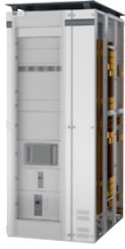
3VA outgoing feeder panels 3NP1 modular installation devices
