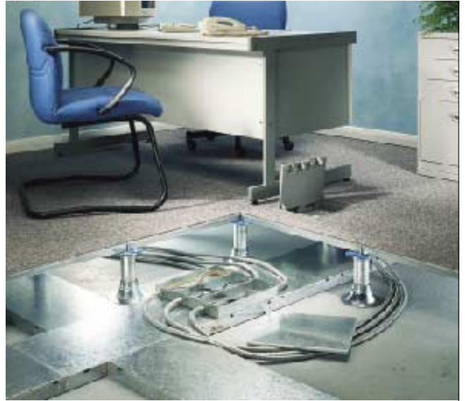
IN-CAVITY FLOOR TRUNKING
