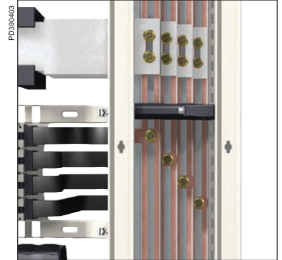
All connection points are directly accessible from the front of the switchboard.
