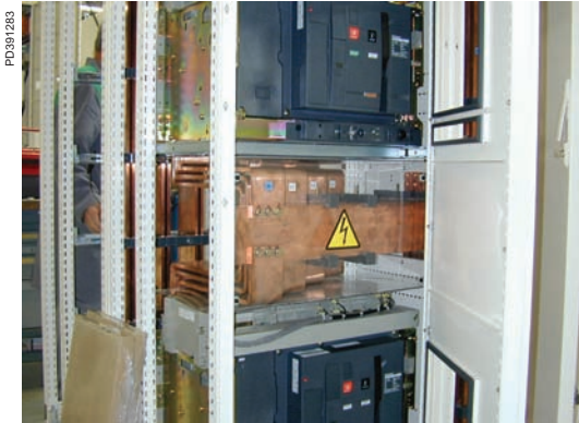
Source changeover system in the same cubicle.
