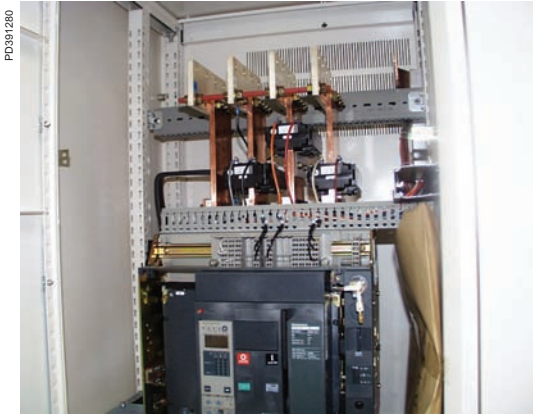
CT on vertical busbars.
