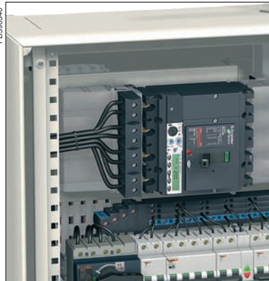
Additional 35 mm 2 blocks installed on the connection between the device and the busbars.
