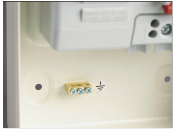
16mm Earth terminating point inside enclosure
